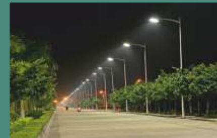
Electric line with Street Light
