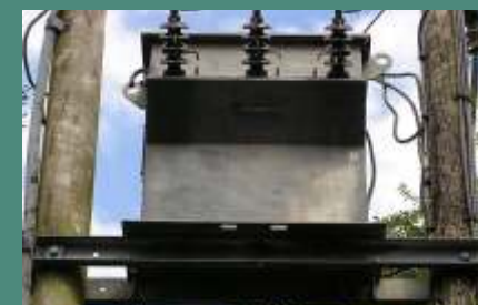
Separate Electric Transformer
